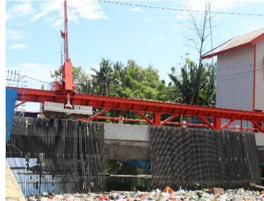
Gambar 3. Pos Pengoperasian Trash rack Kanal Jongaya
